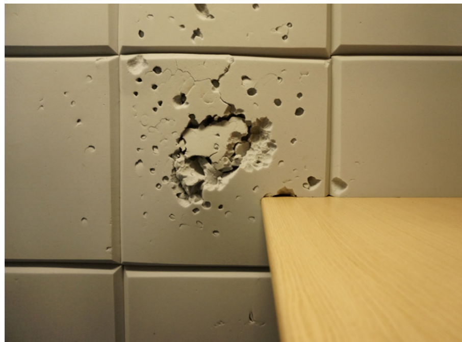
Torn soundproofing in a Cobham AVL studio
